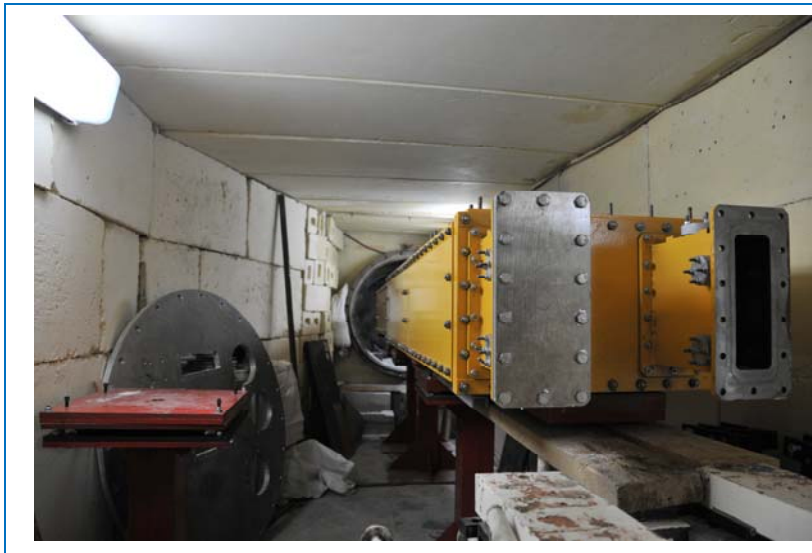
Fig. 12. The head part of the mirror neutron guide installed on beam 6 of the IBR-2 reactor in the framework of the realization of the project of construction of the new DN-6 diffractometer for microsample investigations.
