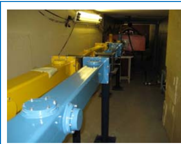
Fig. 4. First sections of the curved neutron guides for EPSILON (yellow) and SKAT (blue).
