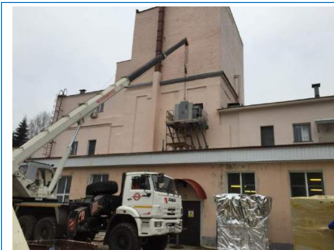
Fig. 27. Lifting of modulators to the accelerator hall through a specially made opening.
