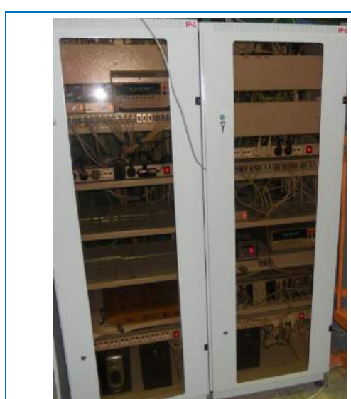
Fig. 59. Control electronic equipment racks for CM-201, CM-202 and KGU.
