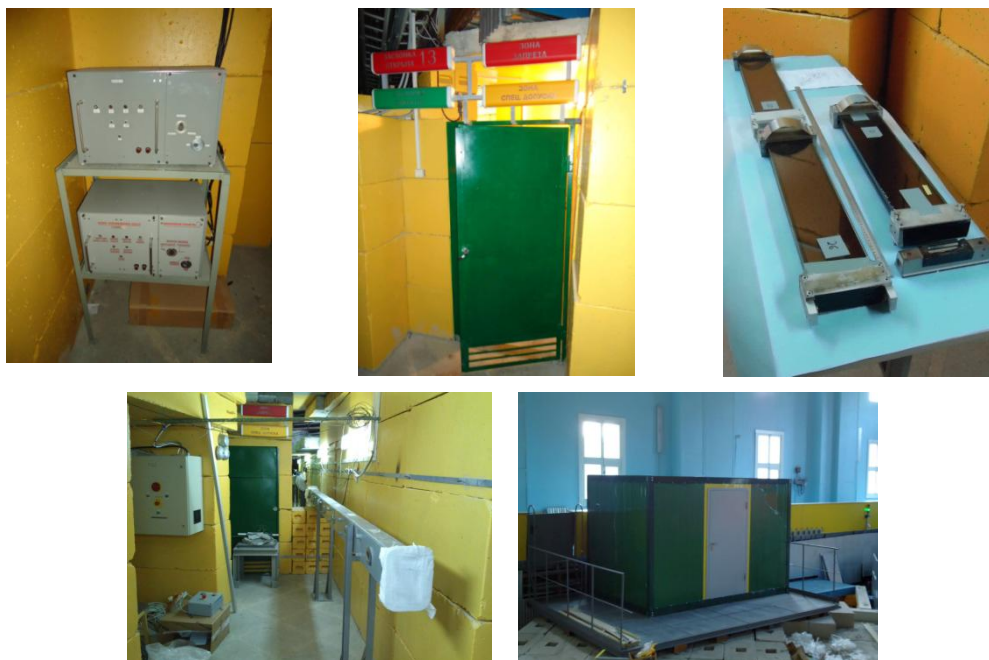
Fig. 22. Fourier-diffractometer FSS on IBR-2 beamline 13 (from top to bottom and from left to right): operational control boxes of a shutter and beam stopper; entrance door to the bunker (beam exit location); glass mirror neutron guide sections before installation in a housing; neutron guide installed in a steel housing and control electronics of the Fourier chopper; experimenter's control cabin mounted on the biological shielding of beamlines № 13-14.
