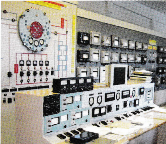
VVR-c control room
